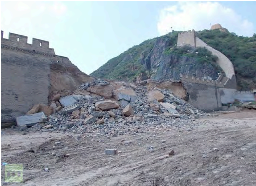
Fig. 4: Wall Collapsed after Heavy Rain, 2013, Hebei Province, China. Source: Autonomous Nonprofit Organization “TV-Novosti”, http://rt.com/art-and-culture/great-wall-china-collapse-355 [accessed 9 December 2013].
